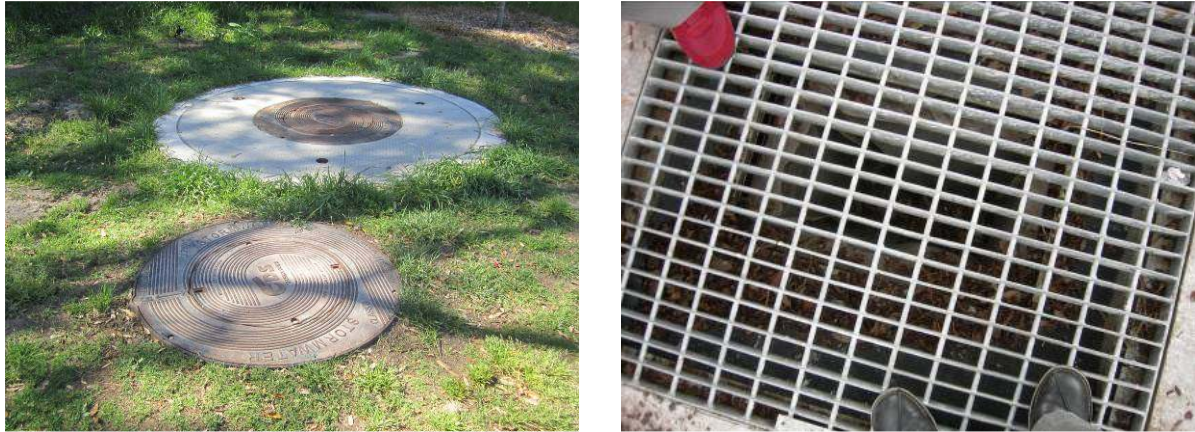
Figure 3: GPT in Centennial Park (left), inlet basket (right) (Photos: Alluvium)
