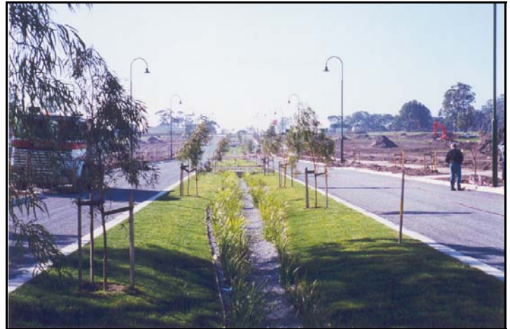
Figure 5 Construction of a Bioretention System in the median strip of a divided street in the Lynbrook Estate for both water quality improvement and flow attenuation.
